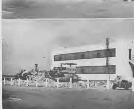
RAZED IN June was the concrete-block Field Engineering Office which was located east of the General Office Building. The 1000-square-foot structure was erected in 1941.
